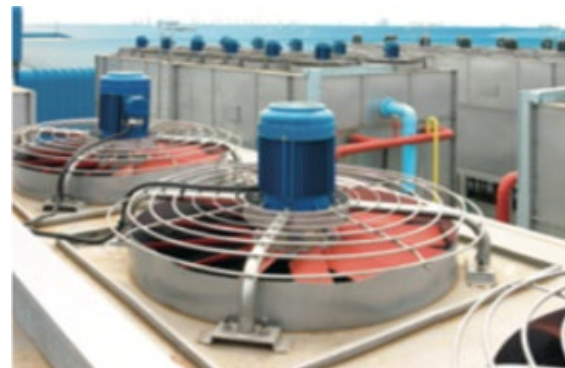
Fan and water pump
